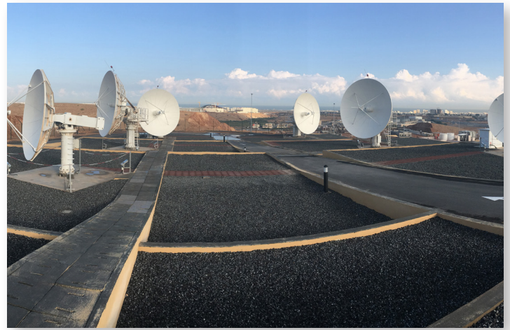
Kratos' state-of-the-art antennas for advanced monitoring.
